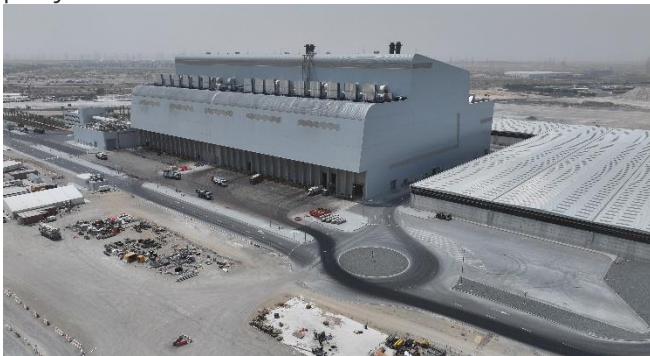
Drone view image of the main plant front elevation taken in June
