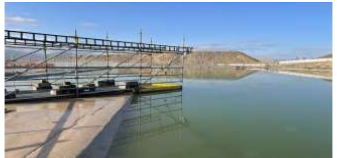
The plant stormwater reservoir did its job, collecting nearly 10,000 cubic metres of rainwater.
