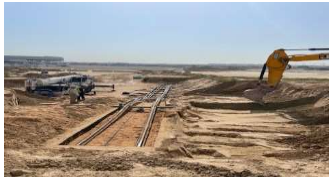
Works to repair the damaged cables were started in the last week of April.
