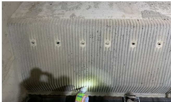
Inspections of the boiler tubes in L11 underway during the outage period.
