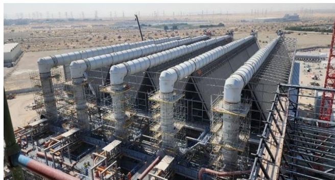
The Air Cooled Condenser units looking south
